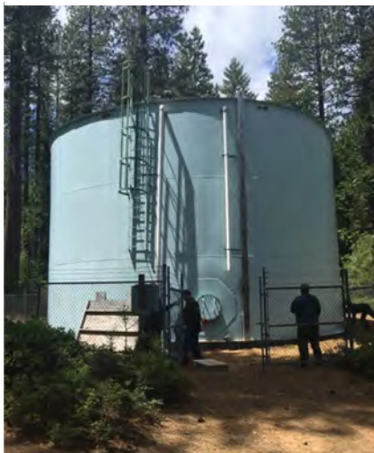
Figure 2-7 - 210,000 gal Storage Tank
