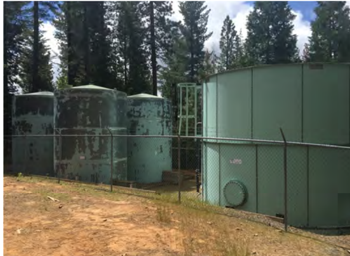
Figure 2-6 - 12,500 gal (4) and 43,000 gal Storage Tanks
